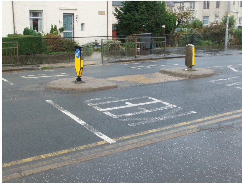
Worn markings at crossing point
